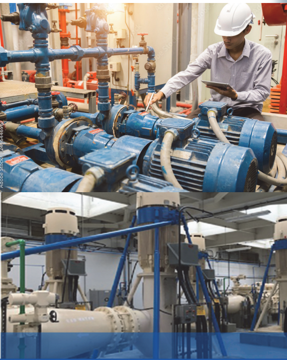
Water pumps benefitting from a Yaskawa U1000 VFD's improved system efficiency.
